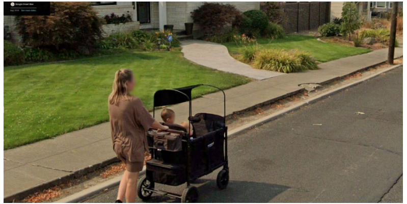
Figure 16. Crumbling Sidewalk, southwest side of Division Street between 7th and 8th Avenues
