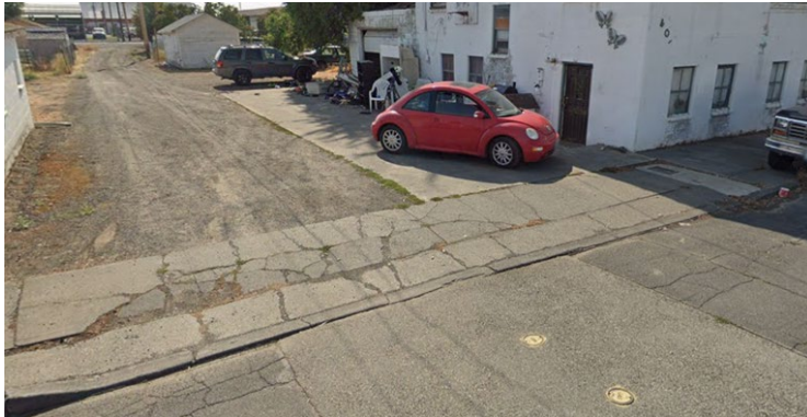
Figure 17. Crumbling Sidewalk, southwest side of Division Street between Birch and Alder Avenues
