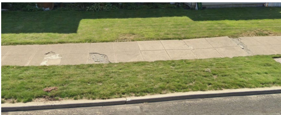
Figure 18. Crumbling Sidewalk, southwest side of Columbia Street between 6th and 7th Streets
