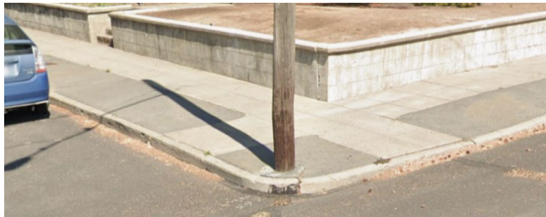
Figure 38. No Curb Ramps on Columbia Street at 3rd Avenue
