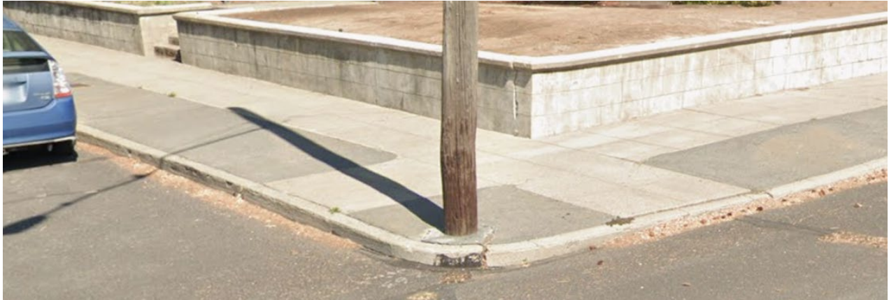
Figure 22. No Curb Ramp at Intersection of W 3rd Street and S Columbia Street
